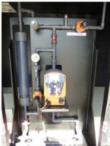
Chemical dosing systems
