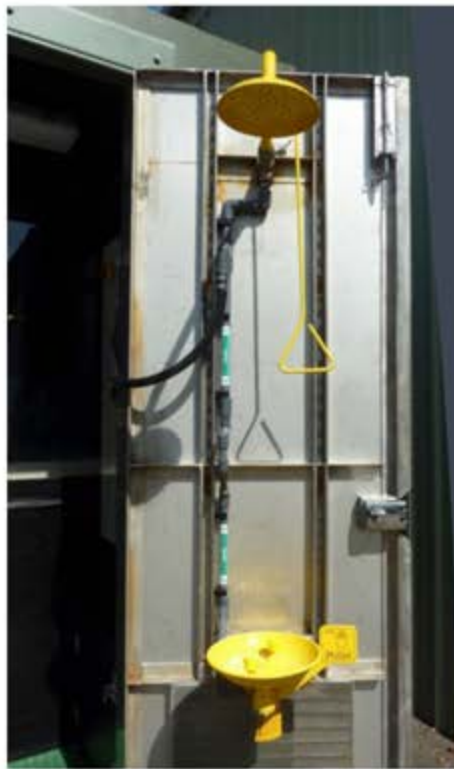
Door mounted safety shower and eye wash.
