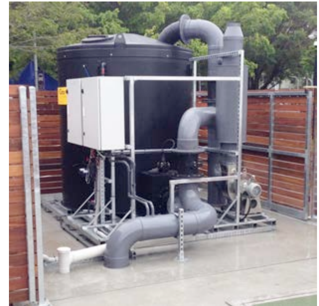
FiltaOdor™ Biofilter installed for Cairns Regional Council WWPS (Waste Water Pump Station)
