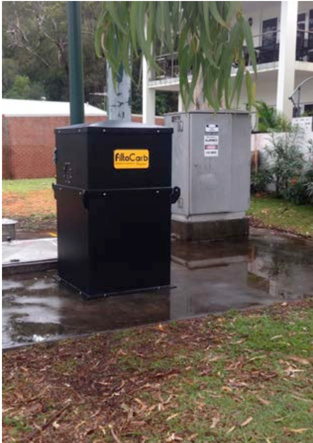
FiltaCarb™ FCC150 cube series filter built for Hunter Water Corporation – Corlette W.W.P.S. (Waste Water Pump Station)
